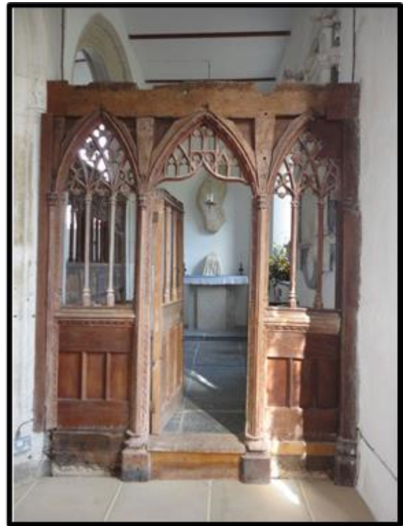
Fig. 303 The screen at Cornworthy showing damage following the loss of the loft and dado panels (RWP Cornworthy DSC04876).
