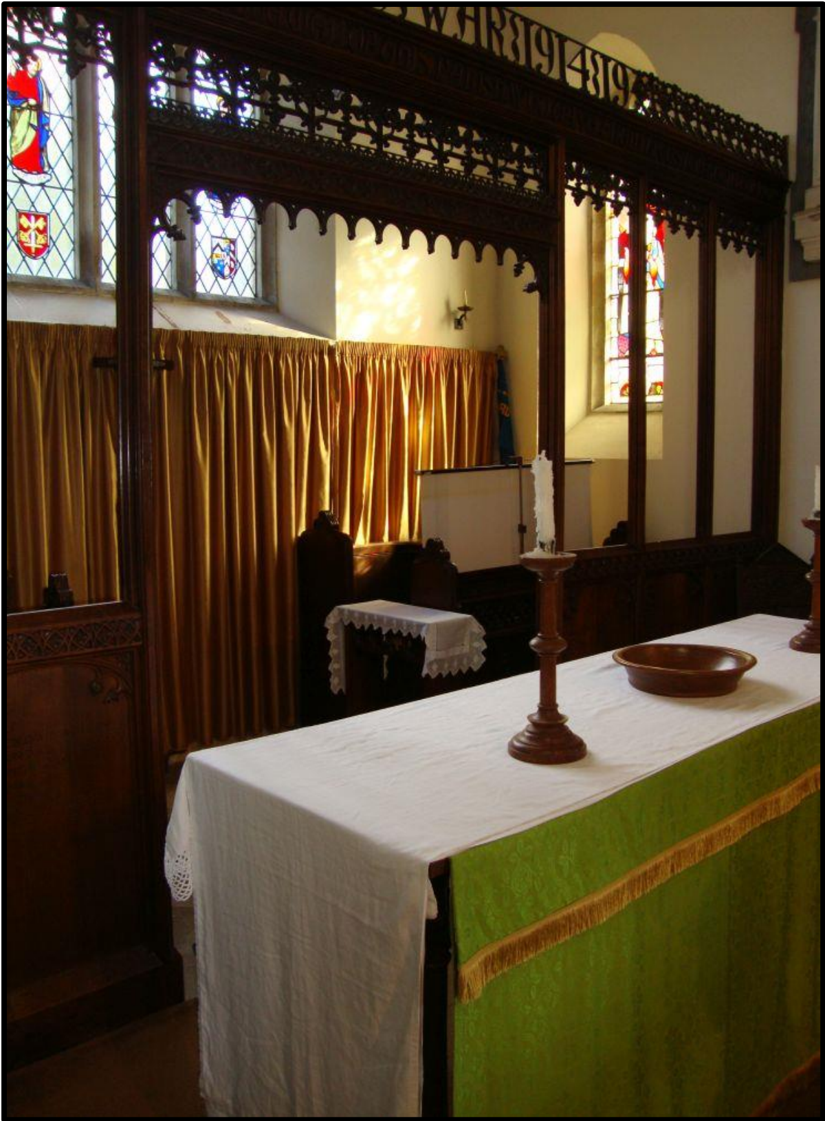
Fig. 47 The rood screen at Sandford, a Great War memorial, as removed out of its historic and liturgical context to the east end of the chancel, creating an awkward and unusable space which is now used for storing lumber (RWP Sandford DSC09380).
