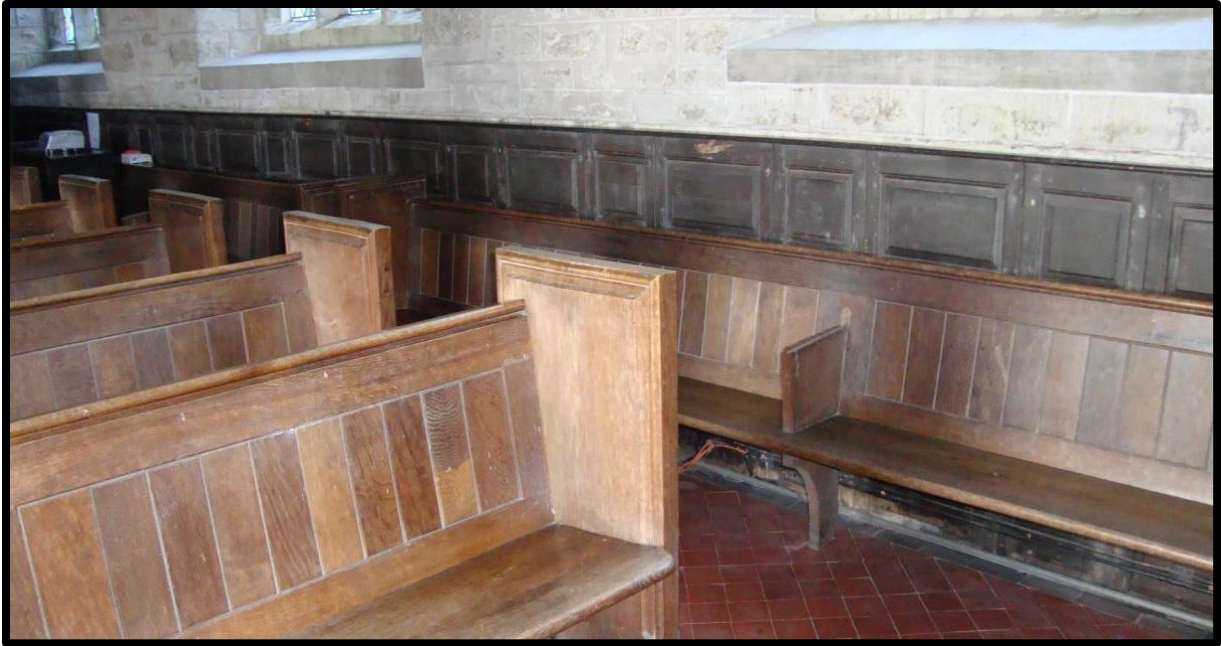
Fig. 82 The remains of the box pews at Bridford, reset as a dado around the walls (RWP Bridford DSC09662).
