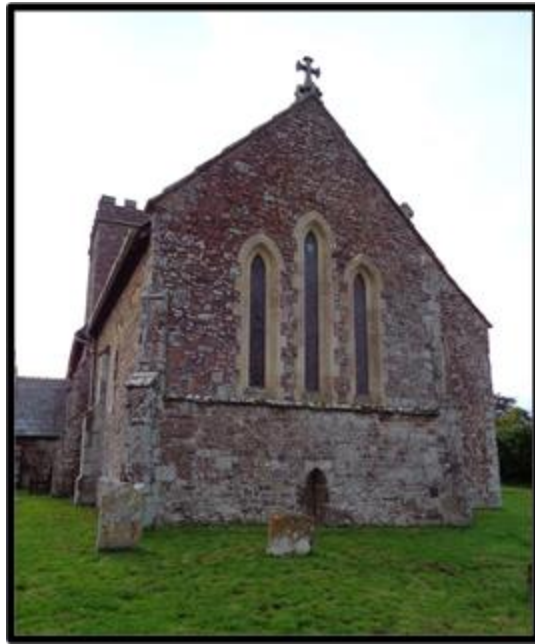
Fig. 288 The window for the former crypt at Stockleigh Pomeroy (RWP Stockleigh Pomeroy DSC00109).
