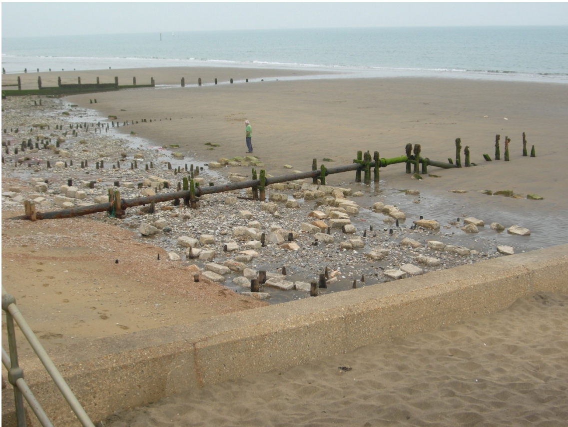
Figure 5.10 Falling beach levels at Yaverland, August 2008 which revealed timber groynes shown on mid-nineteenth century Ordnance Survey mapping but which had not been seen in living memory
