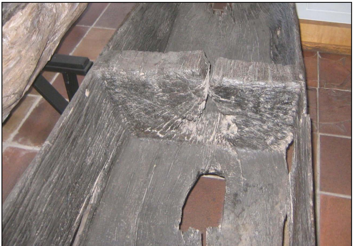
Figure 4.47 Hole cut in the Čelákovice vessel floor just aft of the forward bulkhead.
