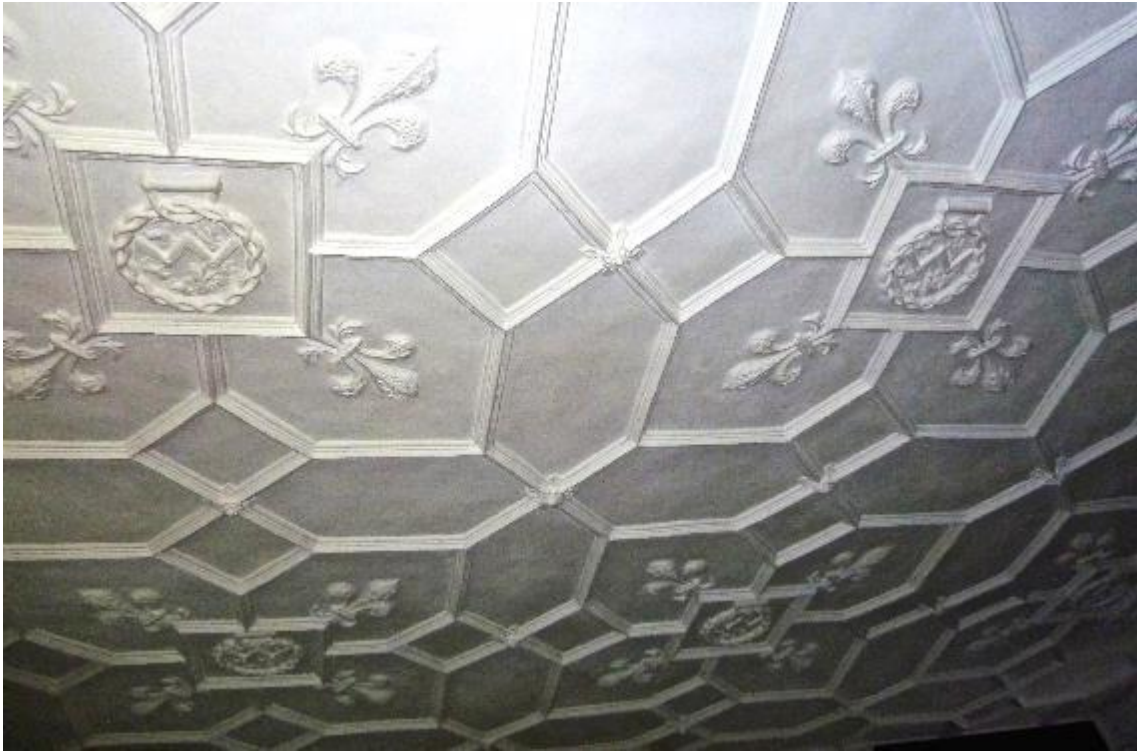
6.23 Ceiling, upper chamber, Orchard Wyndham, Somerset (WS29), [Reproduced with the kind permission of Jenny Chesher].
