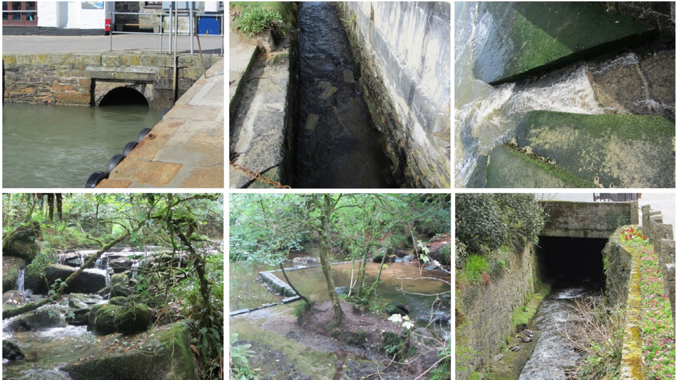
FIGURE A4 Examples of barriers in four streams in south Cornwall. Clockwise from top left: the mouth of the Mevagissey Stream; a canalised section of the Portmellon stream; the mouth of the Portmellon stream; the Polperro flowing through one of several culverts in Polperro village; heavily silted impounded section of the Kennall River at the Kennall Vale gunpowder works; barrier to upstream movement of trout, Kennall Vale.
