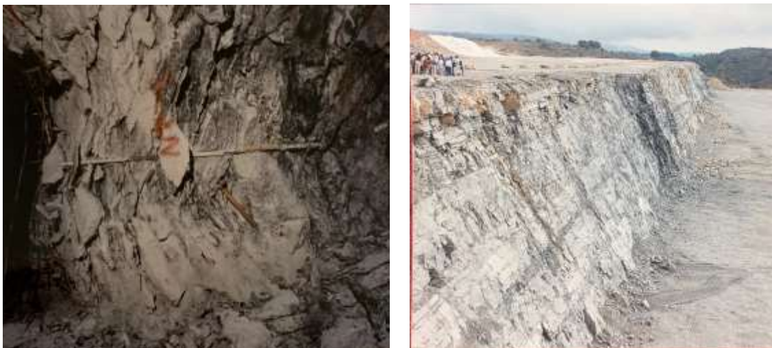
Figure 2. Left: Damaged wall at a crossing section between two temporary mine drifts in talc schist, at 450 m of depth: poor profile due to uncontrolled blasting and texture of the rock mass; half of a 2.5 m long rockbolt is in the plasticized/sheared zone of the pillar (Italy). Right: 18 m high bench in horizontally laminated limestone, careful blasting and scaling (Portugal). (credits Oggeri)
