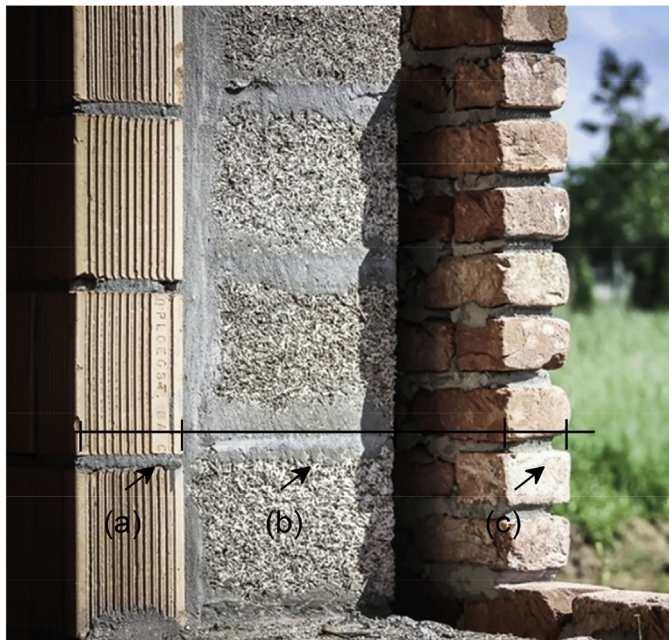
Fig. 5. Illustration of a typical bio-based cavity wall assembly made of hemp concrete. (a) load bearing fired clay blocks, (b) layer of hemp concrete blocks and (c) outer leaf layer of bricks (Courtesy of Isohemp, 2020).
