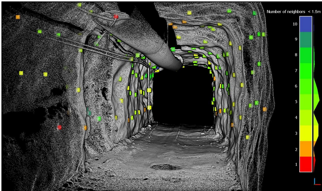
Figure 3-8: A visualisation of the bolt density reporting. The red bolts have less than 1 other bolt within 1.5 meters and have been flagged for further inspection.
