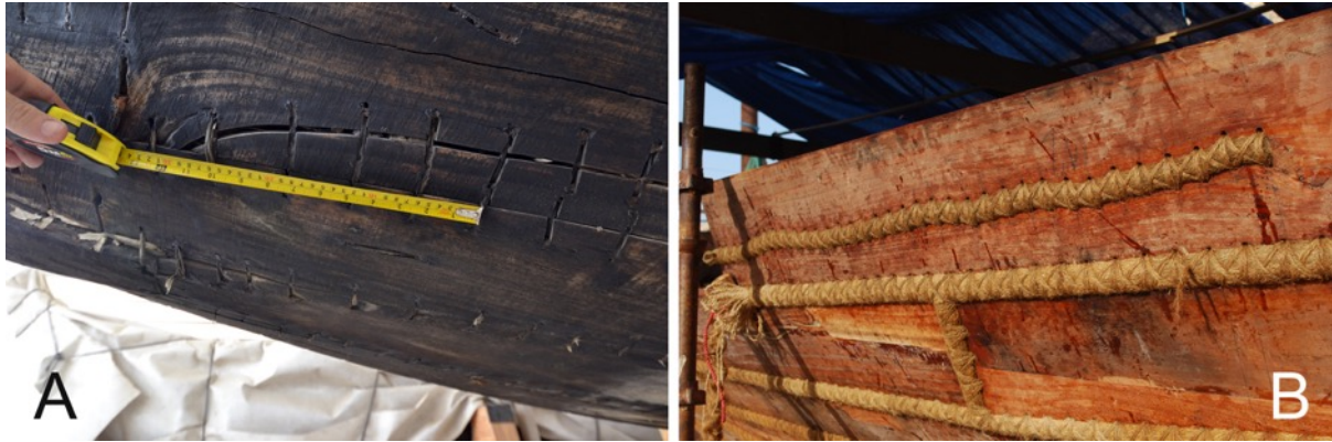
Figure 6.25: A large crack repaired by sewing on QM kettuvallam B (A); and on Jewel of Muscat (B). (Photos: Author)
