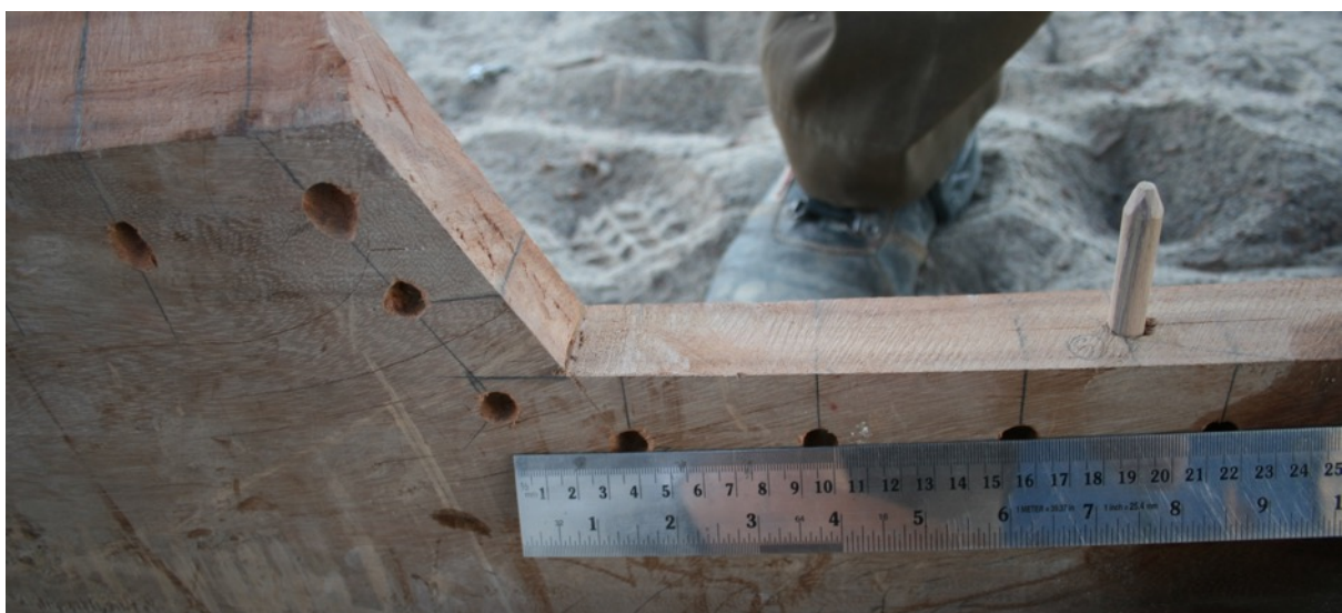
Figure 6.14: Blind dowels used during the construction of Jewel of Muscat . (Photo: Author)
