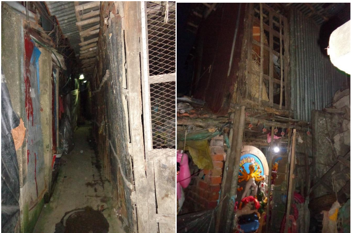
Figure 4.4: Unsteady tin-bamboo structures as the workshop in the deep lanes of Kumartuli (source: author)
