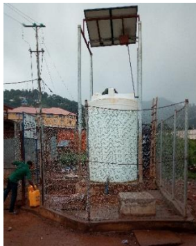
Community installed water tank at Wellington
