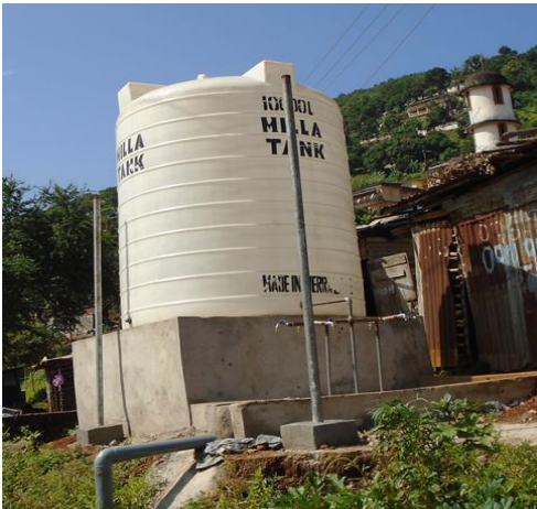
Figure 5. 2 Water provided in 10,000 L tank at Kissy Brook
