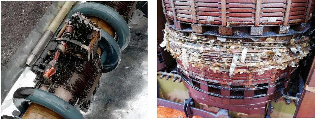
(a) (b) Figure 17: (a) Damaged on-load tap changer and (b) damaged B phase of HV winding.
