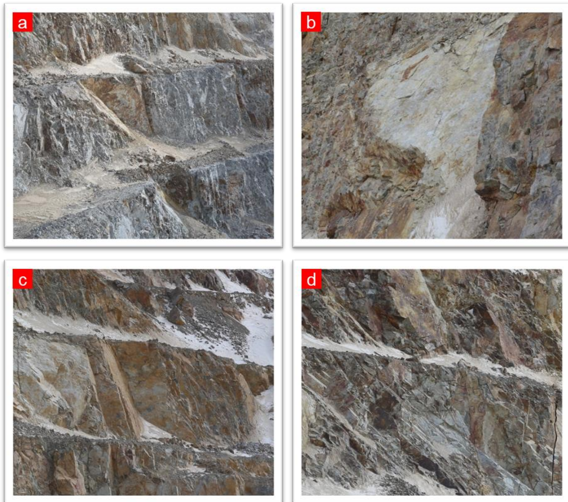
Fig. 6-2. The scar of other bench failures in the west slope, showing the geometric characteristic of failure planes.
