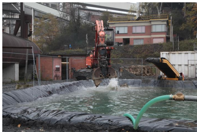
Figure 6. Schemes for alternative feeding of soils into the basin: bucket excavator and conveyor belt (top), pumping of slurry (middle), and picture of the installation (bottom). Capital letters (in squares) are references for the identification of the individual branches of the hydraulic circuits.
