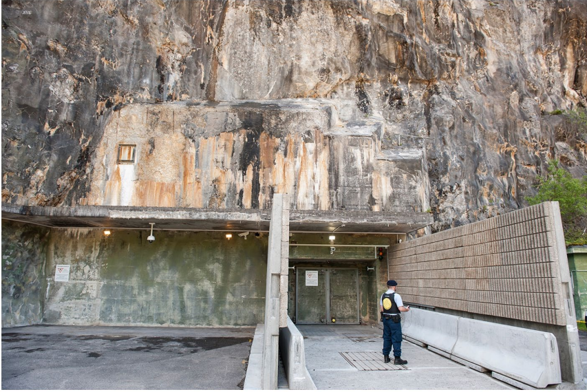
Figure 1. The entrance to one of the two bunkerized data centres operated by the cloud back-up provider Mount10 (pronounced ‘Mountain’), both of which are located in former military bunkers in the Swiss Alps. Mount10’s data bunker complex is known as the ‘Swiss Fort Knox’ (image courtesy of Mount10).
