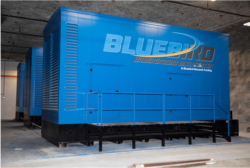
Figure 12. Bluebird Network operates an underground data centre located in a former limestone mine in Missouri. The facility uses 2MW diesel-fuelled generators (pictured above) for its emergency off-grid power supply (image courtesy of Bluebird Network).
