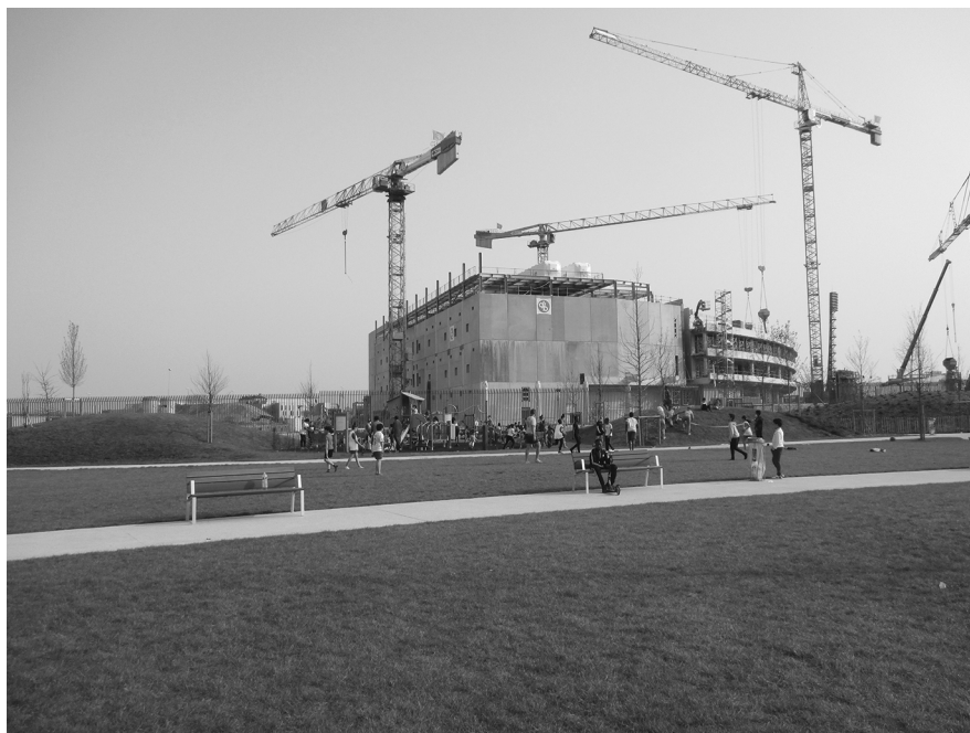
Fig. 4.3: First building (of four) of Interxion's future data centre campus, construction site in La Courmeuve, April 2021. Photo by author.
