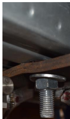
Bolted studs' failure.
