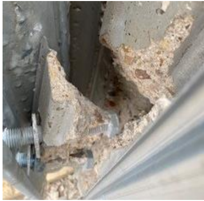
Concrete cone failure.
