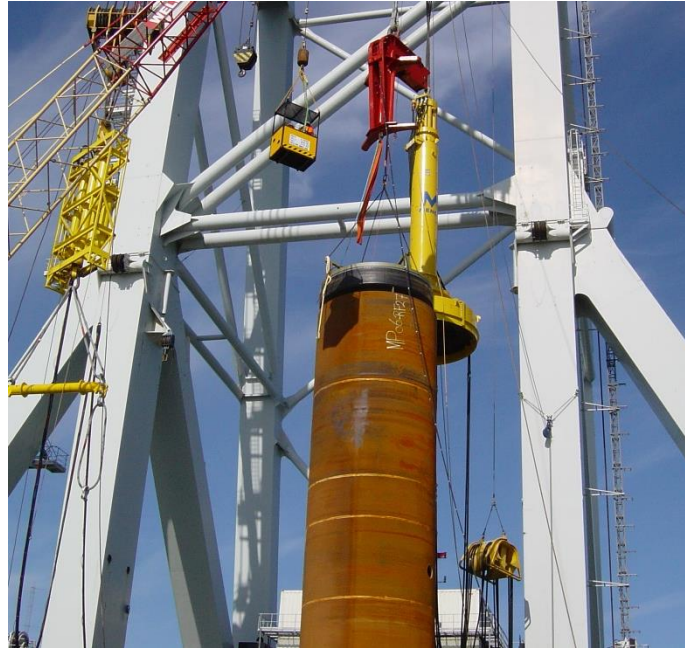
Figure 1-7: Driven monopile (brown cylinder, centre) and piling hammer (yellow unit, top centre)
