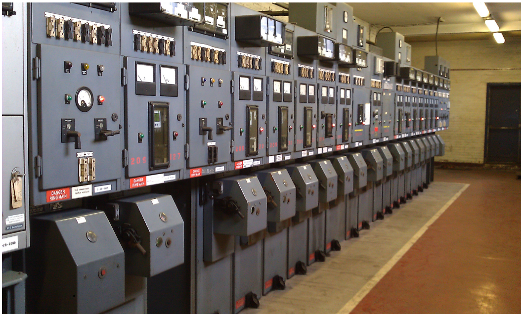
Figure 7.4: 11kV Surface Substation (Three Phase, Triple Pole Switches)
