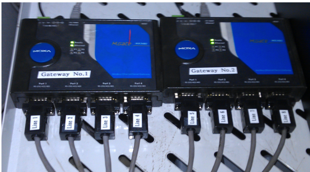
Figure 7.8: Moxa MODBUS Gateways (The 11kV Substation Server)
