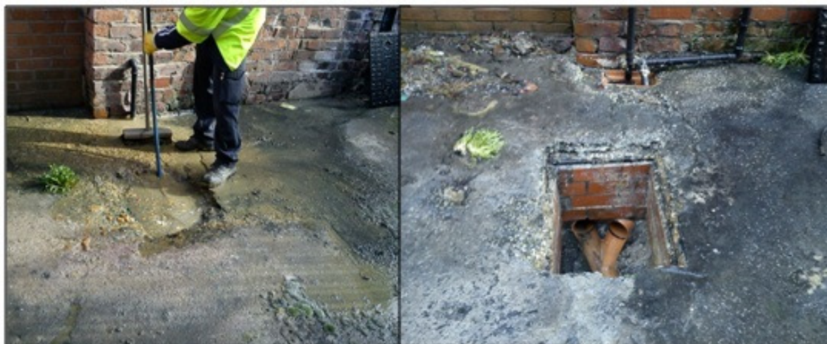
Figure 3-1 Location UU/A - Manhole before and after blockage removal; operative was able to subsequently identify blockage was removed from a private asset
