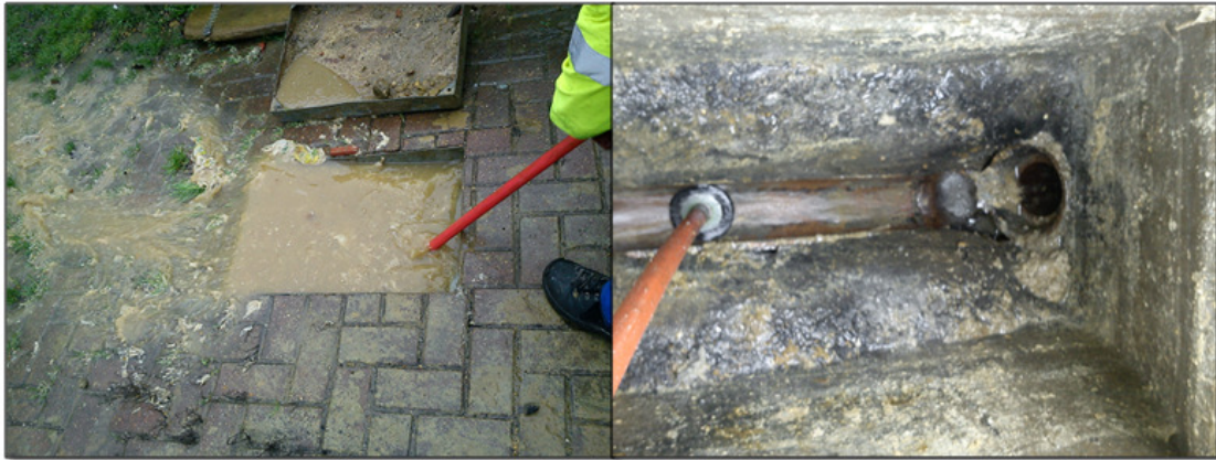
Figure 3-6 Location AW/3 - Blockage removed from an interceptor trap, recorded as 'no cause'
