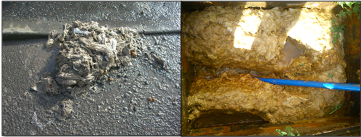
Figure 3-4 (Left) Location NIW/C - Gross non-degradable solids which would be likely to cause a blockage downstream. (Right) Location STW/E - Degradable solids which can be removed with the flow and so do not require removal from the system
