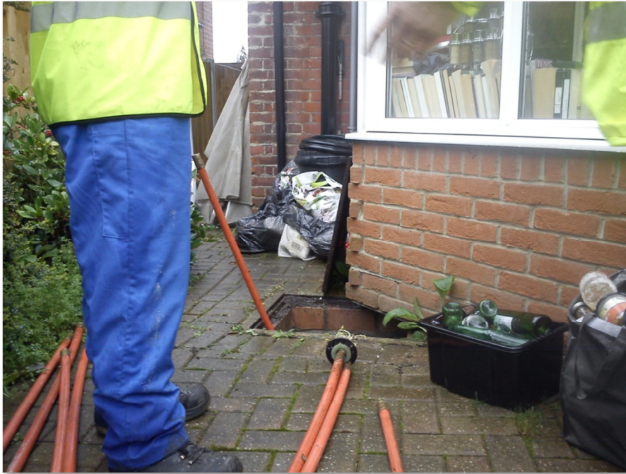
Figure 3-5 Location AW/2 - Blockage on a section 24 sewer to rear of property; cleared with rods as could not access with jetter
