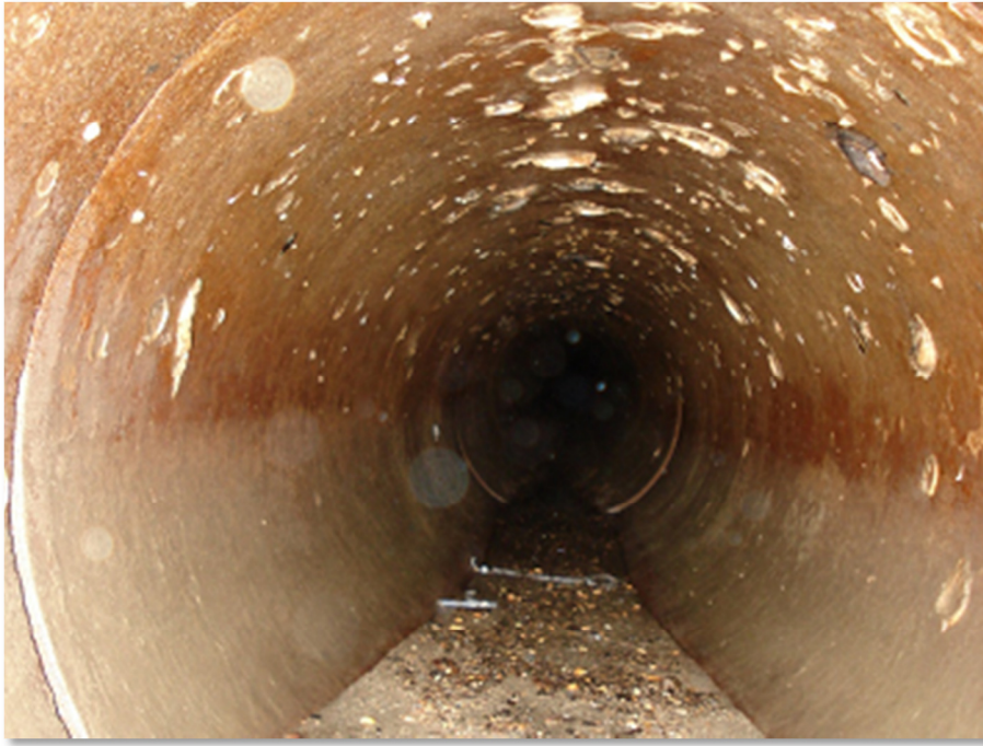
Figure 2-6 Sediment and grit deposited on the pipe invert (image courtesy of WRc)
