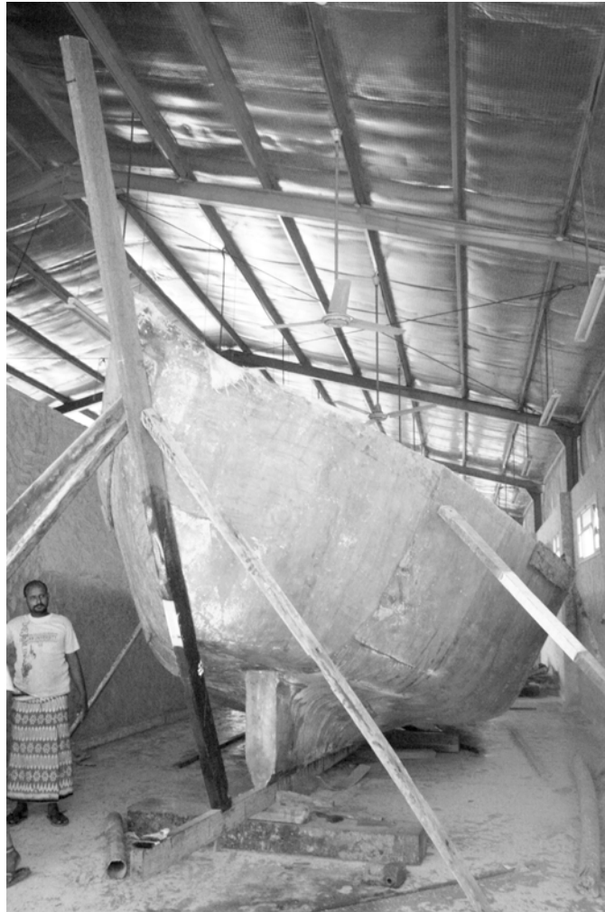
Figure 9: A fibreglass galbah under construction at al-Ṣalīf. The hull form retains that of the wooden ʿobrī (MARES/J.P. Cooper).
