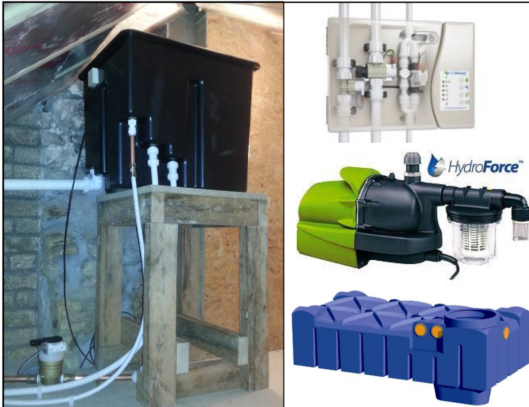
Figure 5.3.2 – RWH components (clockwise): 1) Photo of Header Tank & Refresh Water Meter (WM3); 2) System Controller; 3) System pump; 4) 5,000l Tank
