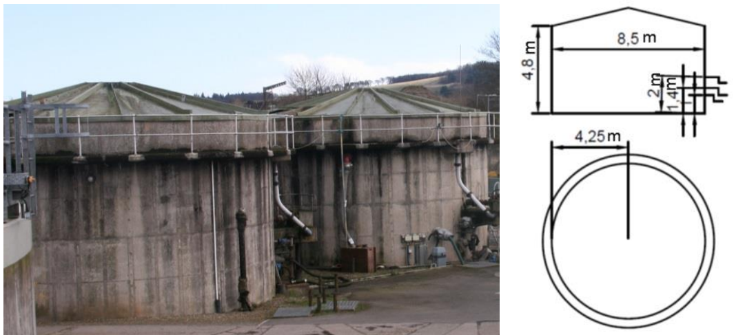
Figure 3-23: Left to right sludge holding tank (in some documents referred as sludge holding tank 1), sludge dewatering tank (in some documents referred as sludge holding tank 2), and longitudinal and plan view of the sludge dewatering/holding tanks; dimensions in meters
