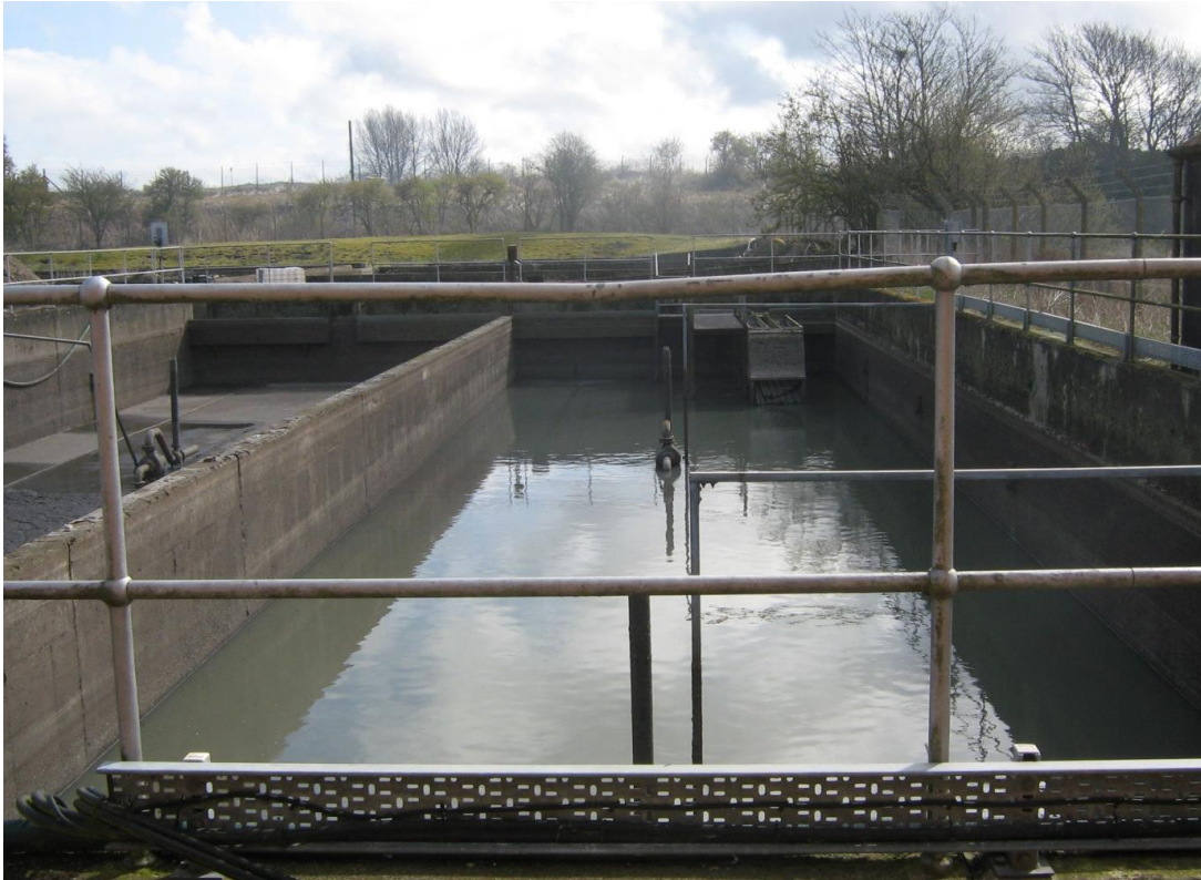
Figure 3-4: Onsite storm tanks at Cupar WWTP
