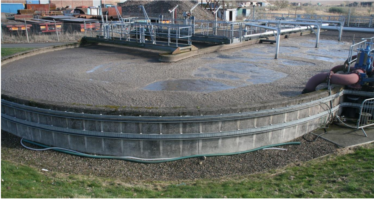
Figure 3-11: Oxidation ditch at Cupar WWTP
