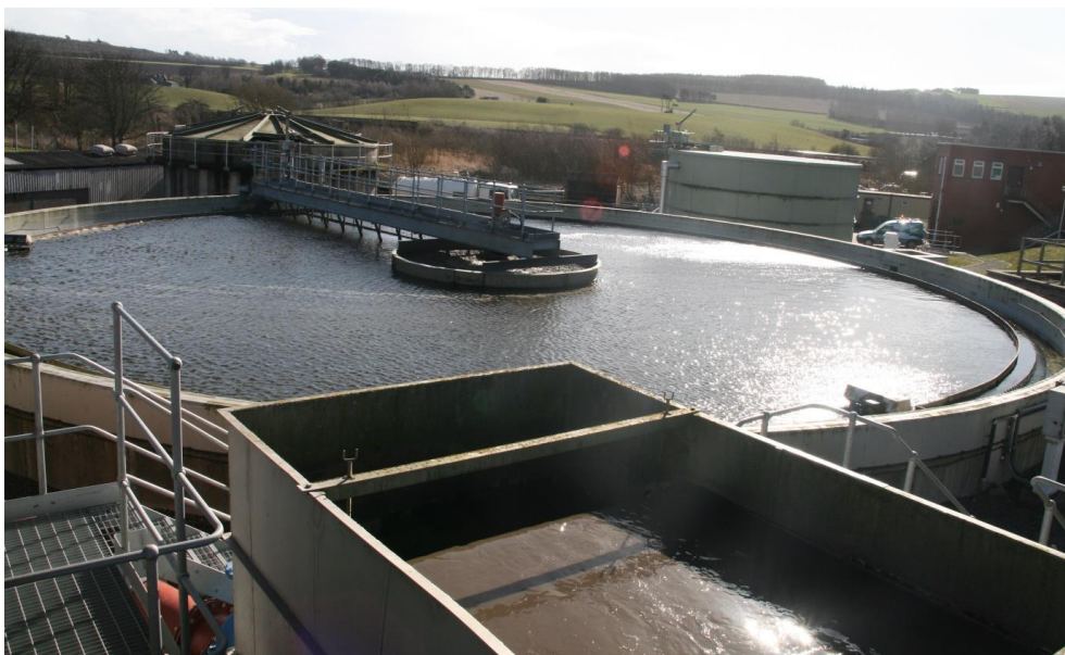
Figure 3-21: One of the final settlement tanks at Cupar WWTP
