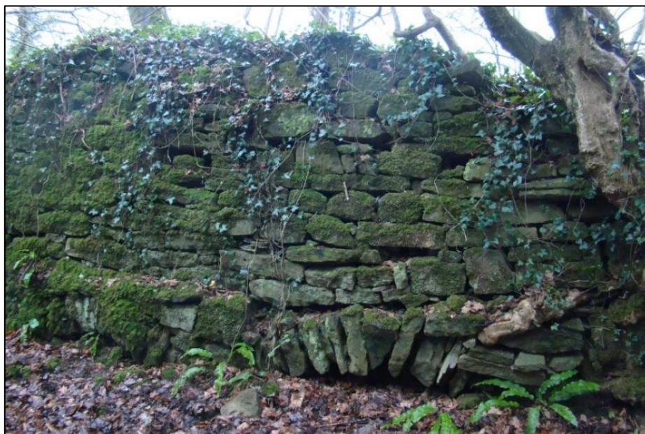
Figure 7.28: Extant section of precinct wall, with the top of buried arch visible (Source: author).
