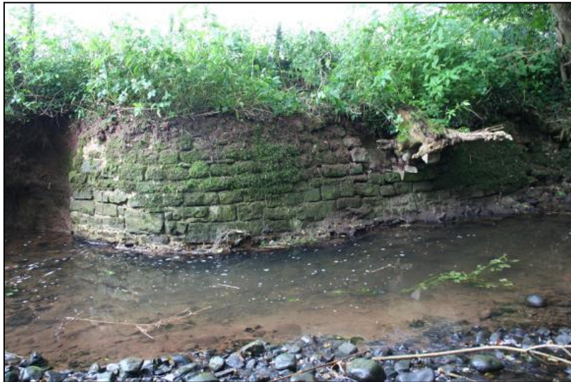
Figure 9.27: Canalised section of Dowlais Brook forming part of the precinct boundary (Source: Standing, undated, www.monasticdave.wordpress.com ).
