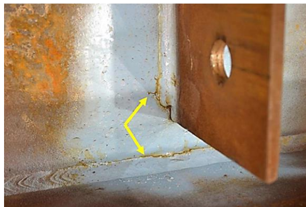
Figure 2.11 Example of web gap cracking resulting from distortion (Dexter & Ocel 2013).
