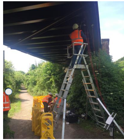
Figure 5.16 A team member installing strain sensors on the girder G2 of the bridge.
