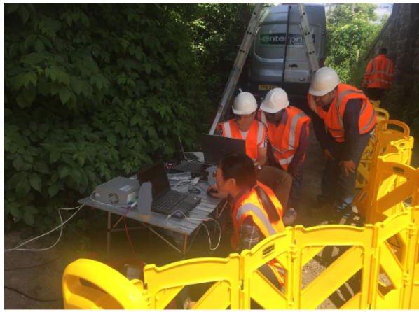
Figure 5.15 Equipment used during the monitoring event.
