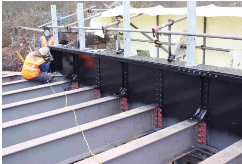
Figure 5.9 Photo of connecting main girder to cross beams using double L angles (WSR).
