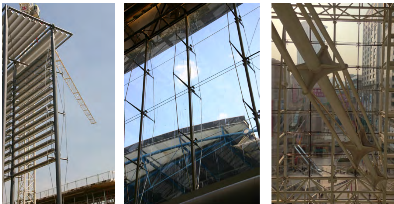
Figure 15. Prestressed stayed columns in practice. Left to right: an example as a slender support for a façade in Chiswick Park, West London; a set of roof supports in the former Eurostar terminal in Waterloo Station in Central London; an example in a shopping mall in Dalian, China. Photographs courtesy of Dr Daisuke Saito and Dr Jialiang Yu.
